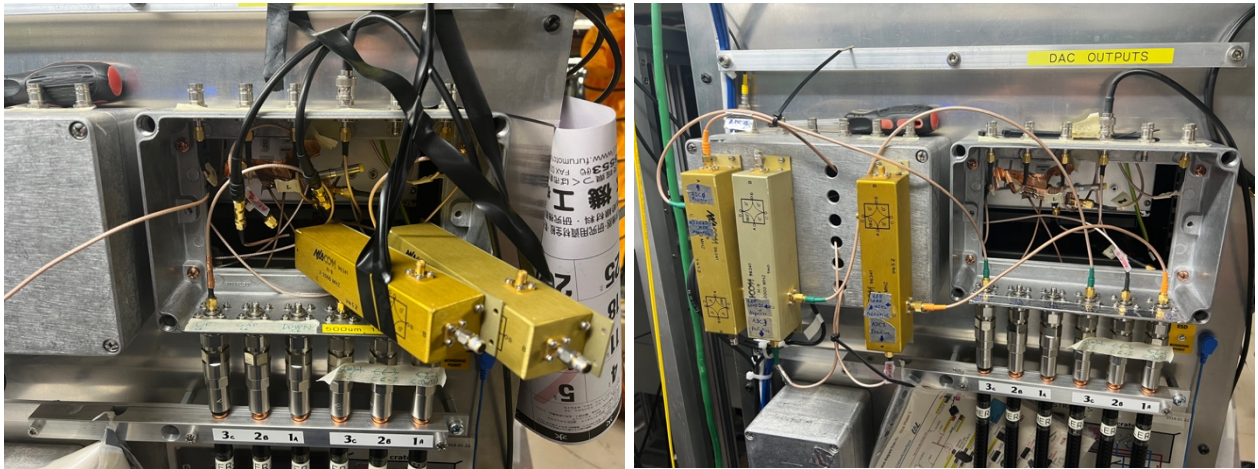
Figure 9 e-Hut inverter configuration before (left) and after access day
